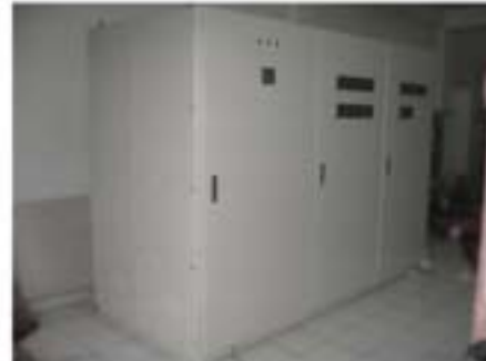
Low Voltage Panel
